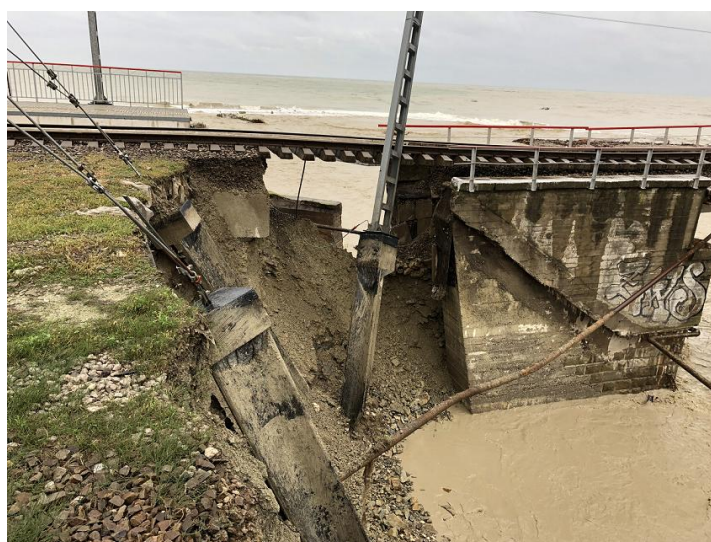
Figure 6. Scour of the bridge over the Makopse River in Tuapse Region due to heavy rains on October 24-25, 2018, which caused mud floods (Source: Russian Railways)
