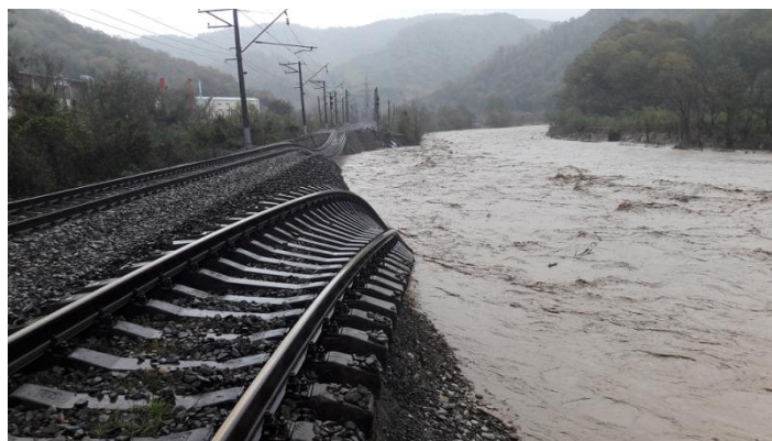
Figure 5. A crash of railway tracks in Tuapse Region due to heavy rains and mud floods along the Tuapsinka River in October 2018 (Source: Russian Railways)
