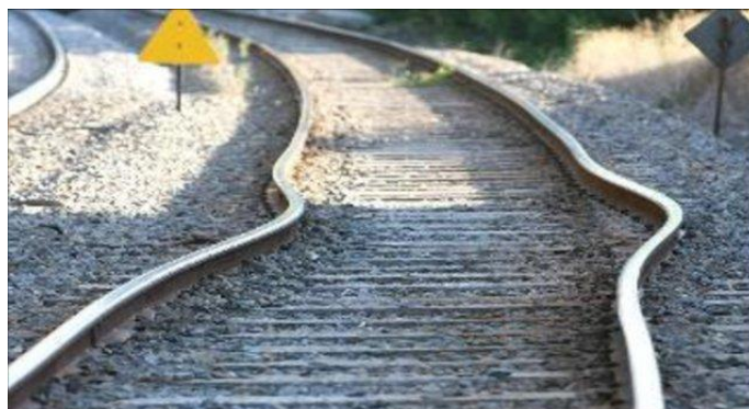
Figure 1. Rail track buckling in Australia (Mandal, Lees, 2016)
