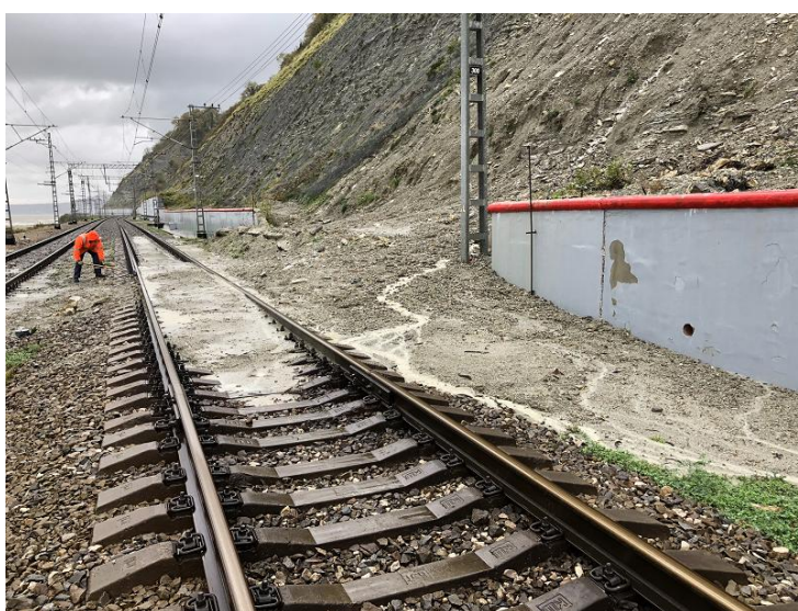
Figure 7. Landslide on the railway tracks in Tuapse Region due to heavy rains in October 2018 (Source: Russian Railways)
