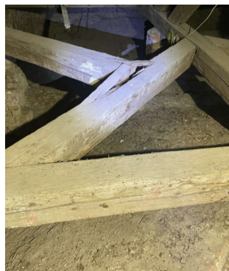
Fig. 3 Element Tear-Out Due to Improperly Constructed Joint.
