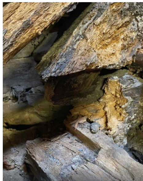
Fig. 2 Damage to a Rafter's is Foot and Beam Due to Moisture and Wood-Decaying Fungi.
