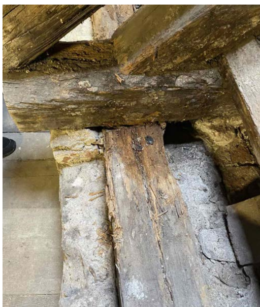
Fig. 1 Impact of moisture on a beam in a roof truss structure
