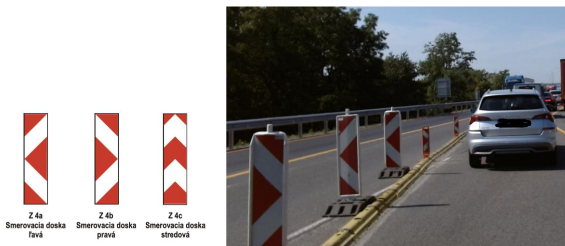
Figure 7: Example of incorrect usage of temporary road signs.
