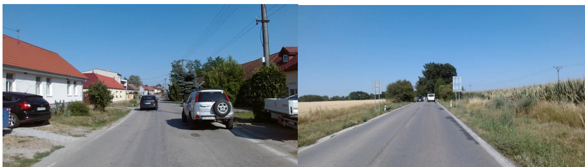
Figure 3: Driving lanes marking not present or almost invisible.
