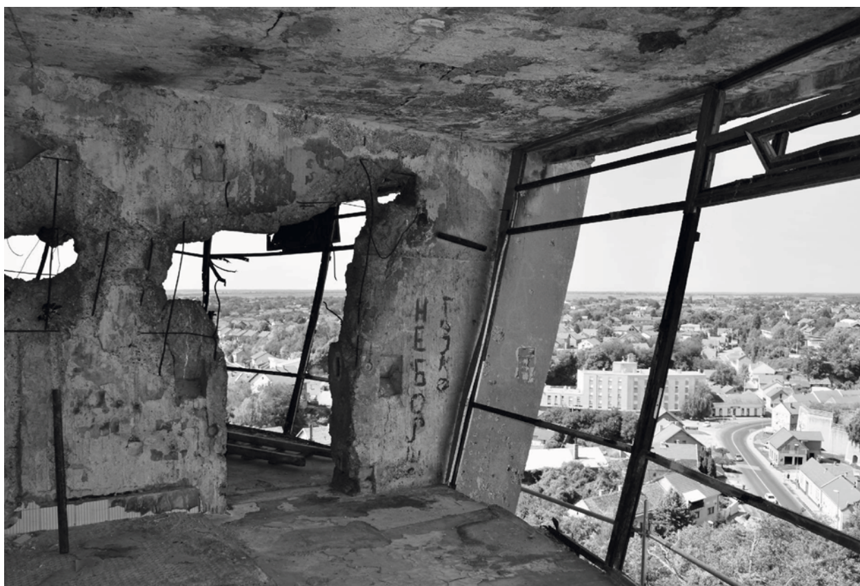
III. 3. Damage to Water Tower, photograph taken before the reconstruction work began. Author: Tena Knezevic, source: personal archive of the author, Antonio Nevescanin
