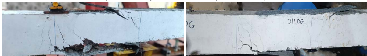
c) Concrete Cover Separation (O2L3G, O1LDG and O1LDL).
