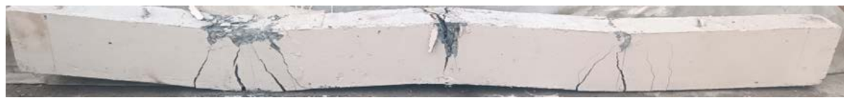
a) Flexural Mode of Failure (CB).
