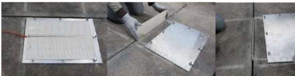
Fig. 23: Instrumented plate installation at the Federal Aviation Administration (FAA) National Airport Pavement Test Facility (NAPTF) in Atlantic City, New Jersey, USA. Source: Grellet et al. [57].
