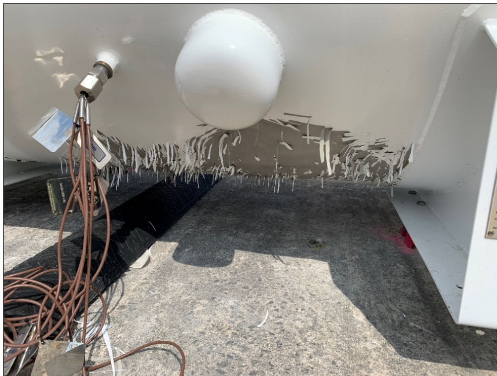
Figure 10 The paint peeling from the underside of the tank.
