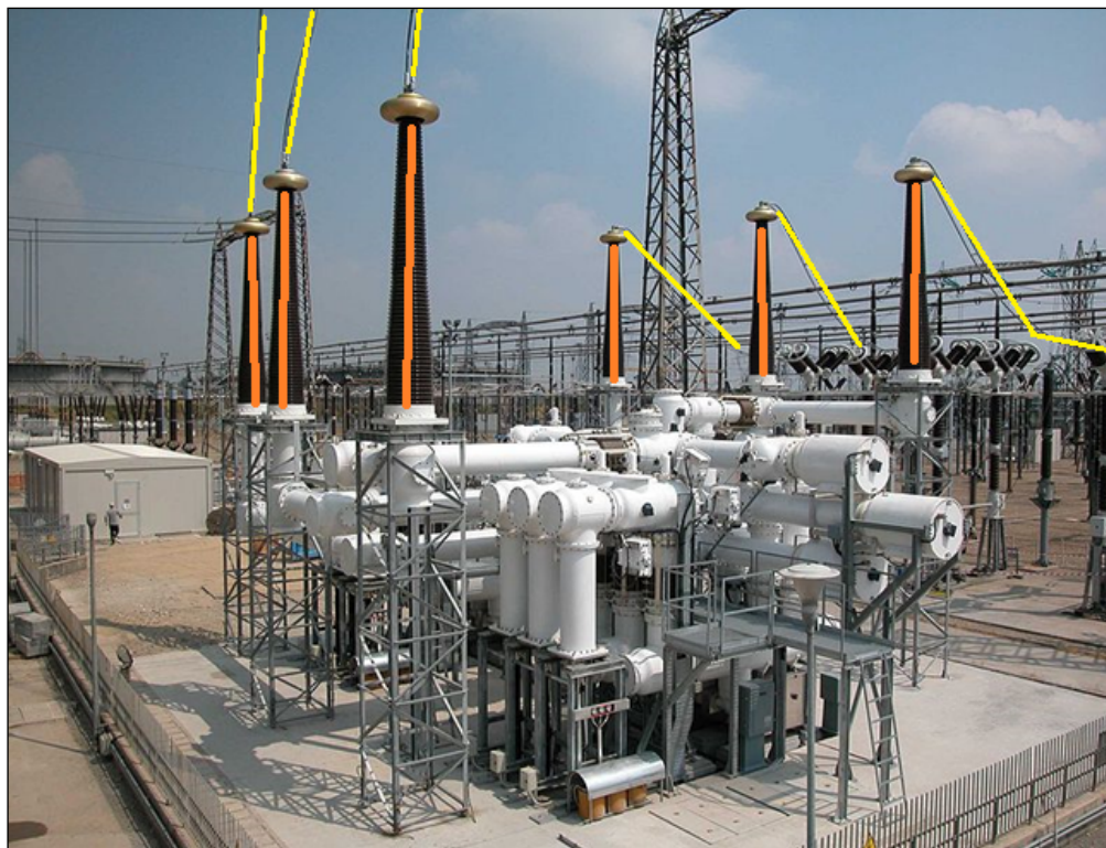
Figure 8 400 kV gas-insulated switchgear (foreground) with six (vertical) GIS-AIS transition bays. Ignition sources from tracking (orange) and corona discharge (yellow) are highlighted. Notable is the lack of sources at lower levels. Source Dingy, CC BY 4.0 via Wikimedia Commons.
