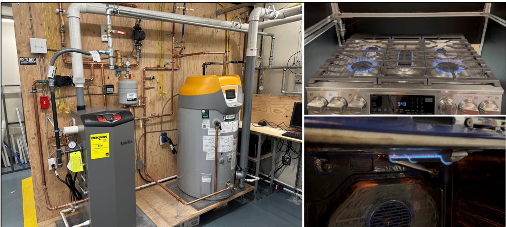
Figure 3 Space heating boiler, storage water heater, and residential stove/oven for HBNG fuel testing.
