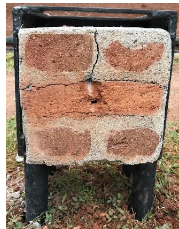
Figure 4.7: Damage Pattern on the MB2 Block
