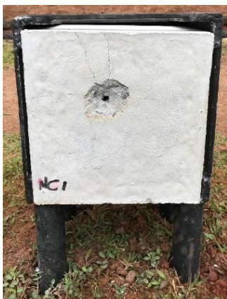
Figure 4.5: Damage Pattern on the NC1 Block
