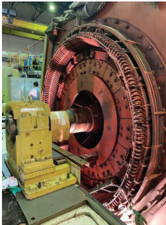
Figure 2 – 20 MW Generator in Sapugaskanda Power Station
