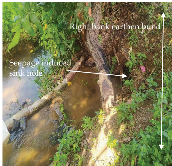
Figure 4 - A Seepage Location at Tissa Wewa
