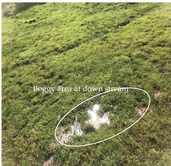
Figure 10 - Present Day Seepage at Vendarasankulam Reservoir
