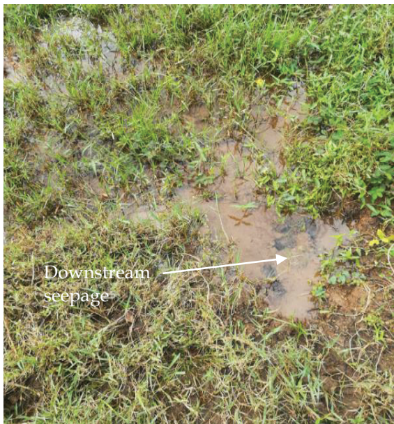
Figure 6 - Seepage in Parakrama Samudra
