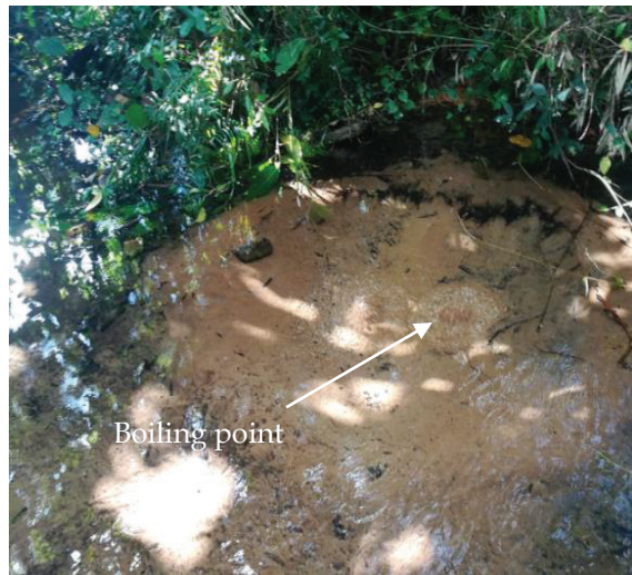
Figure 7 - Seepage Induced Boiling point in Girithale Tank
