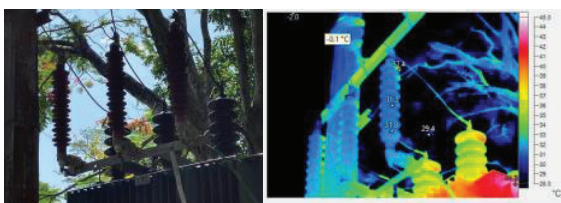
Figure 1 – Photograph of Surge Arresters Connected to a 33 kV Transformer (Left) and Its Thermal Image (Right)
