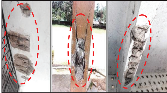
Figure 10 – Defective Structural Elements in an Old School Building
