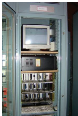
Figure 3 - DAQ Installed in a Power Station
