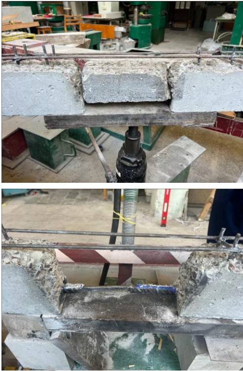
Fig. 5. Overview of the damaged region of the RC beam
