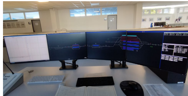
Fig 4. Dispatcher Workstation Equipped with ESA 44 Interlocking, Including a Remotely Controlled Line since 2024
