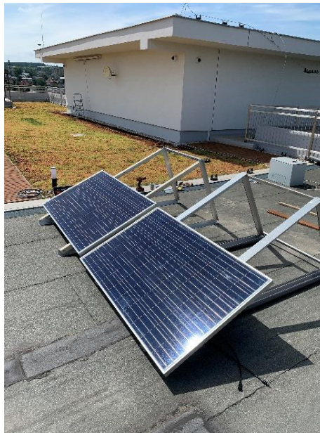
Figure 2: Installed PV panels
