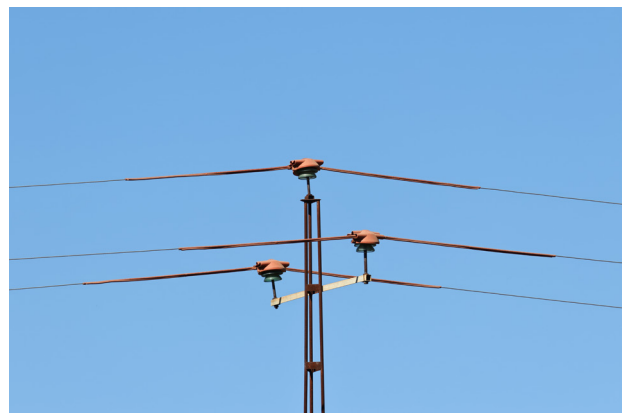
Fig. 3. Bird-safe utility pole after retrofitting to prevent bird electrocution in the study area (© Rafael Hernández).
