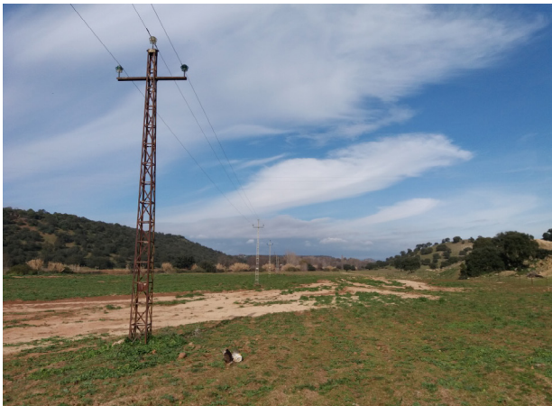
Fig. 1. Landscape of the study area with the power line prior to retrofitting; note the electrocuted bird of prey on the ground (© Manuel Rodríguez).
