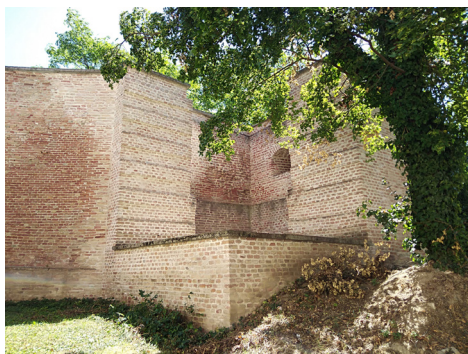
Fig. 1 Picture of the ruin of interest of Trnava's fortified southeastern tower in its actual state in 2021. The point of view is northwest of the interior of the fortification.
