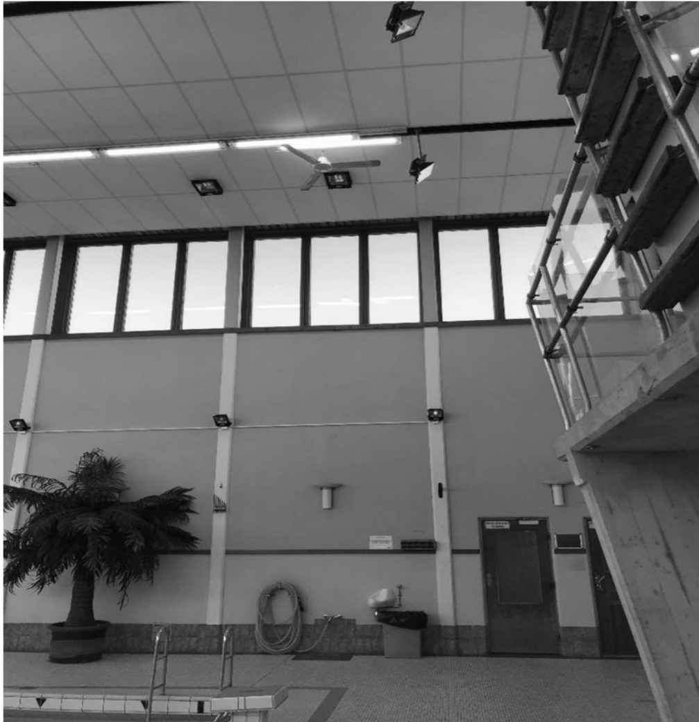
Figure 4 – The photo shows blue light lamps in the bigger pool hall.
