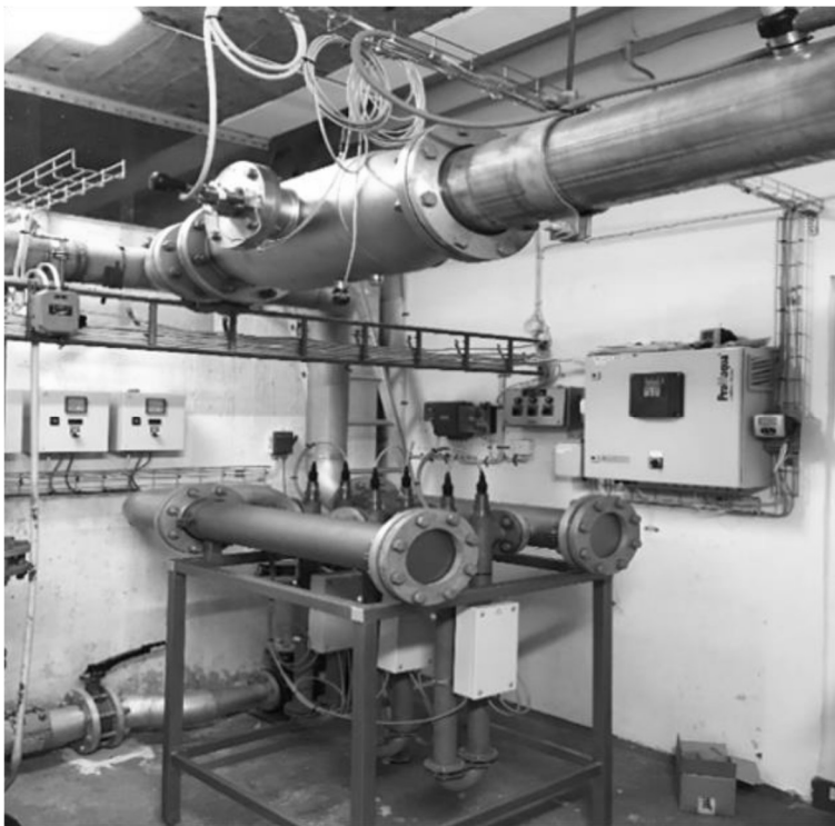
Figure 2 – This picture shows the AOT devices for photocatalysis installed in the treatment plant of Västertorp aquatic center.
