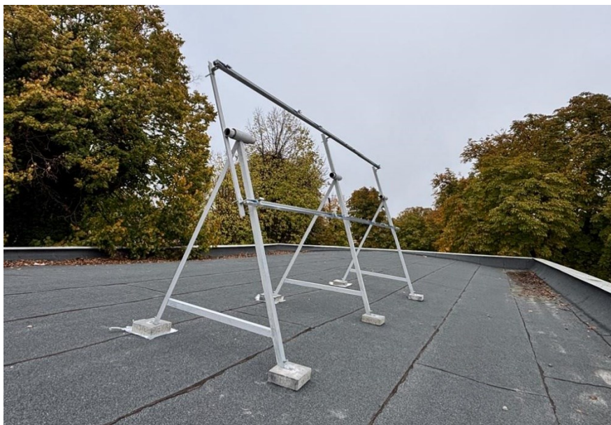
Fig. 6 - Mounting structure of photovoltaic modules with one-axis pivot bar
