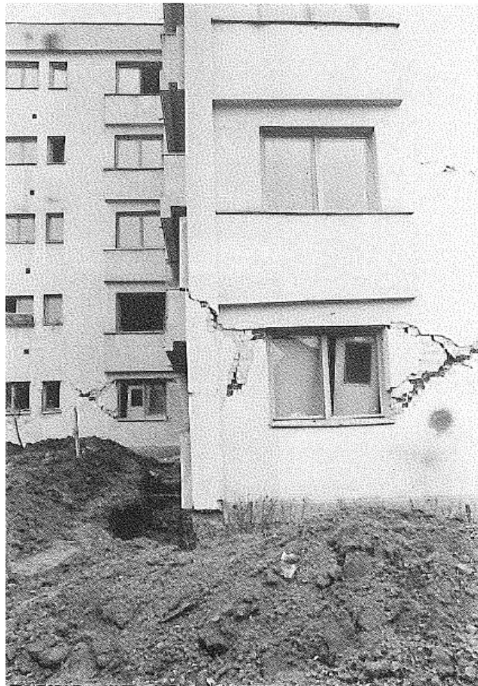
Fig. 3.3 - GF+4 Masonry Buildings Severely Affected by the March 4, 1977 Vrancea Earthquake [8]
