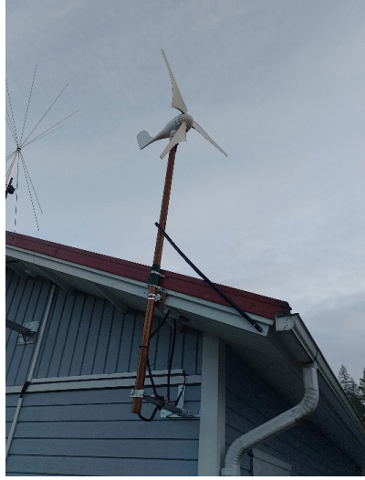
Fig. 1. The wind turbine installation. The crossbeam shown in the picture prevents lateral movement and vibration of the wind turbine mast. The crossbeam was not included in the original design, but after initial experience, it proved necessary. The MPPT is located under the eaves, protected from moisture, while the other electronics are housed in a heated building. The MPPT cannot be installed inside the building, as the cable length would be too long in that case.
