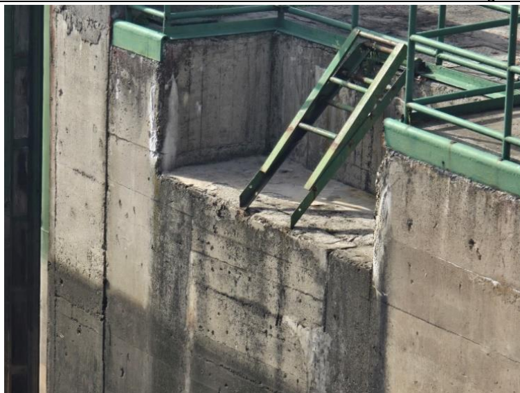
Fig. 1. Structure D, lock wall, carbonation (source: own photo)
