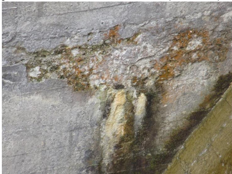
Fig. 3. Structure A, overflow, carbonation and erosion (source: own photo)
