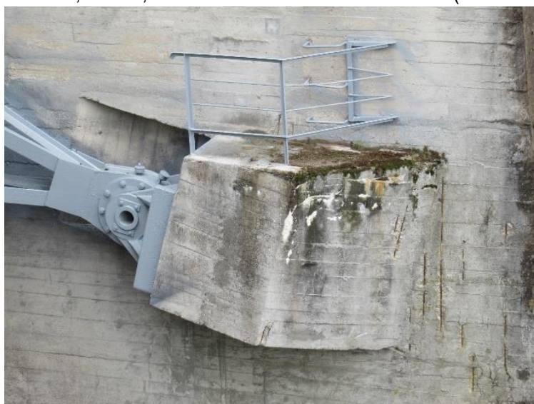
Fig. 5. Structure E, lock wall, corrosion and visible reinforcement (source: own photo)
