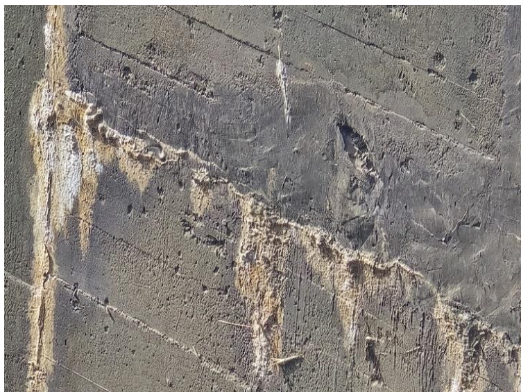
Fig. 2. Structure E, weir, carbonation and leaks (source: own photo)
