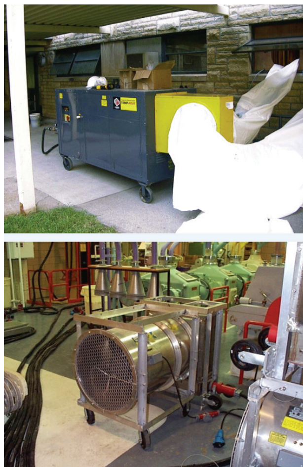
Figure 6. A portable heat-treatment device for delivering hot air into a flourmill from outdoors to control insects (top), and a hot-air blower operating inside a mill that is plumbed into the building's steam.
