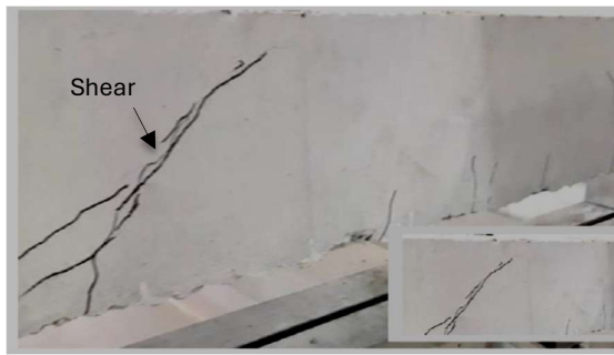
(a) RC beam without steel fibers (B-0): Shear Failure
