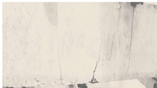
(e) Beam with mixed steel fiber (BM-1.05): Flexural Failure
