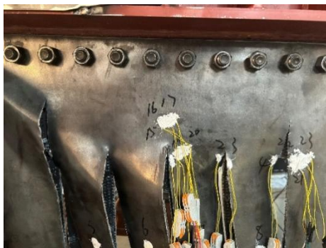
e) Cracks in steel plate
