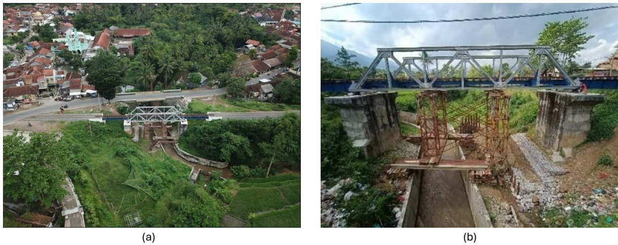
Figure 2: (a) Aerial view of the bridge, (b) Steel structure of the bridge
