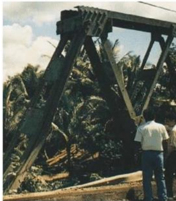
Figure 4: The diagonal member at the end was struck by a vehicle
