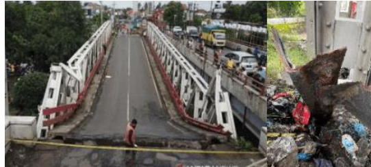
Figure 3: Rembun Bridge after collapsing due to severe corrosion on the bottom chord (right)
