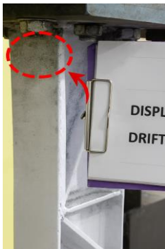
Figure 13(m), Yield condition: paint flaking observed on the flange (specimen LL-4, 6B Cycle).
