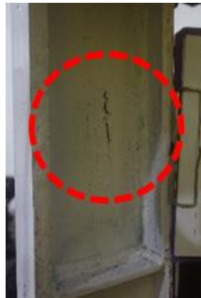
Figure 13(e), Ultimate condition: extensive paint flaking observed on both web and flange sections (specimen LL-1, 8A Cycle).
