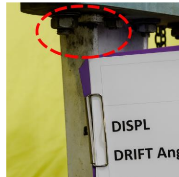
Figure 13(o), Failure condition: fracture at the top weld location (specimen LL-4, 8A Cycle).
