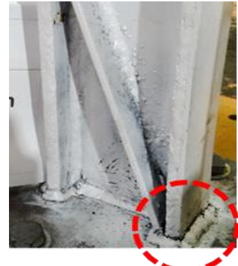
Figure 13(l), Failure condition: fracture at weld location (specimen LL-3, 8A Cycle).
