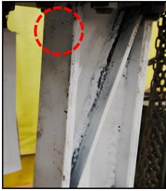
Figure 13(j), Yield condition: paint flaking observed at the stiffener-adjacent flange with minor flaking in the web region (specimen LL-3, 6B Cycle).
