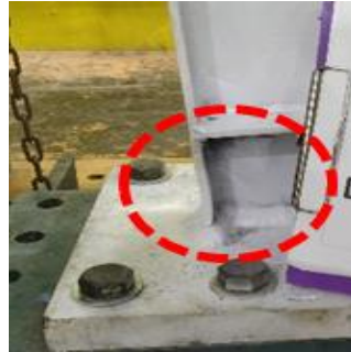
Figure 13(b), Ultimate condition: flange buckling observed at both top and bottom flange regions (specimen LL-0, 10A Cycle).
