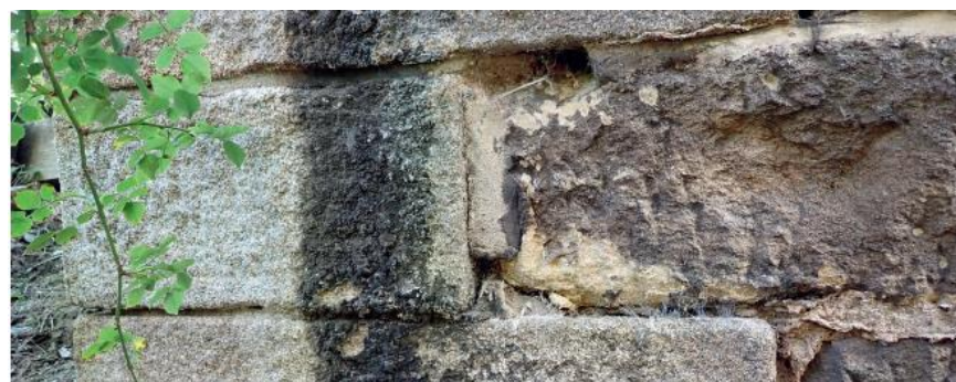
Figure 11: Viaduct near Ratboř – degradation of sandstone blocks and fallen jointing
