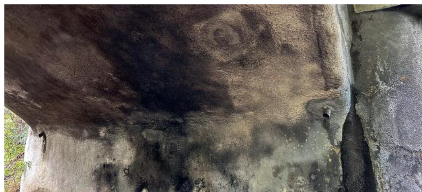
Figure 10: Bridge over the Ohře River in Bohušovice – moisture retention with shotcrete and leaks through shotcrete
