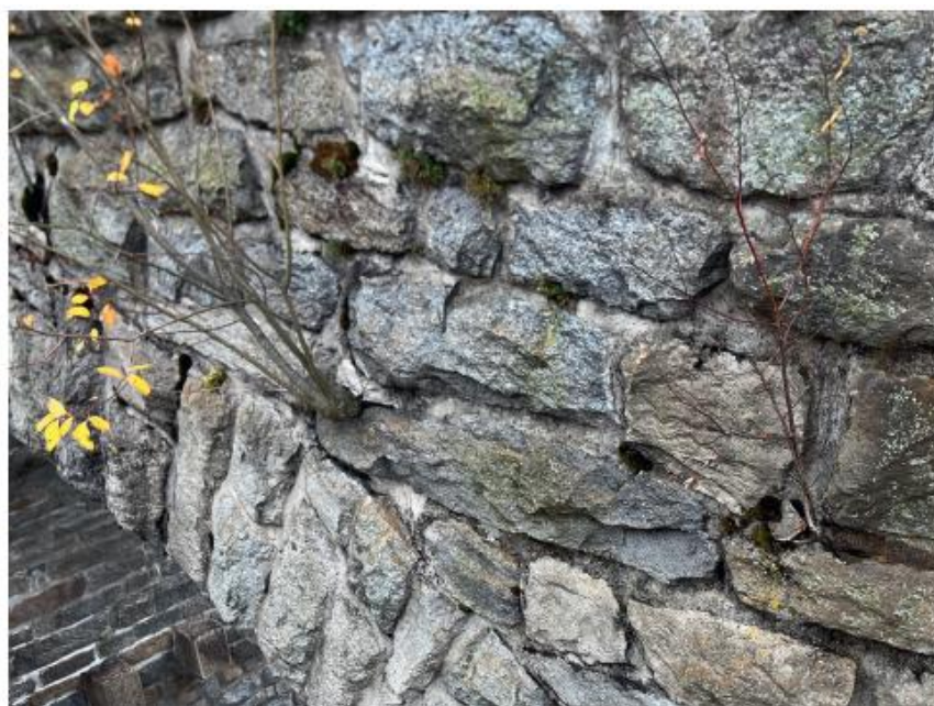
Figure 9: Milevsko Viaduct - vegetation growing through the structure
