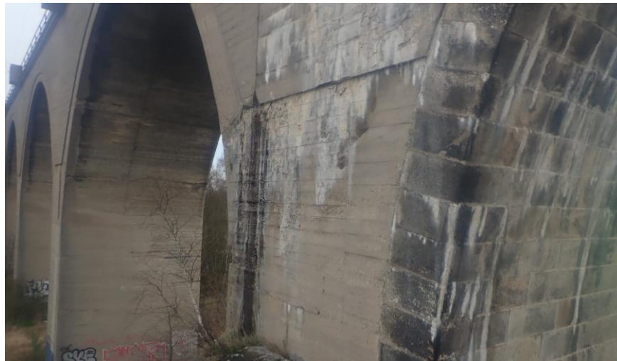
Figure 12: Cheb Viaduct – Degradation and leaching at the joint between the original stone structure and the newer reinforced concrete structure
