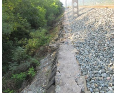
Fig. 7: Geosynthetic clay liner length is insufficient.
