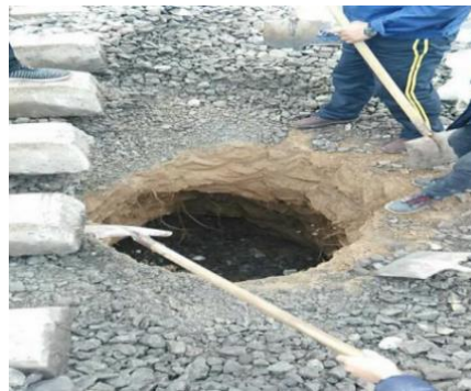
Fig.8 There is a hidden kiln under the subgrade.
