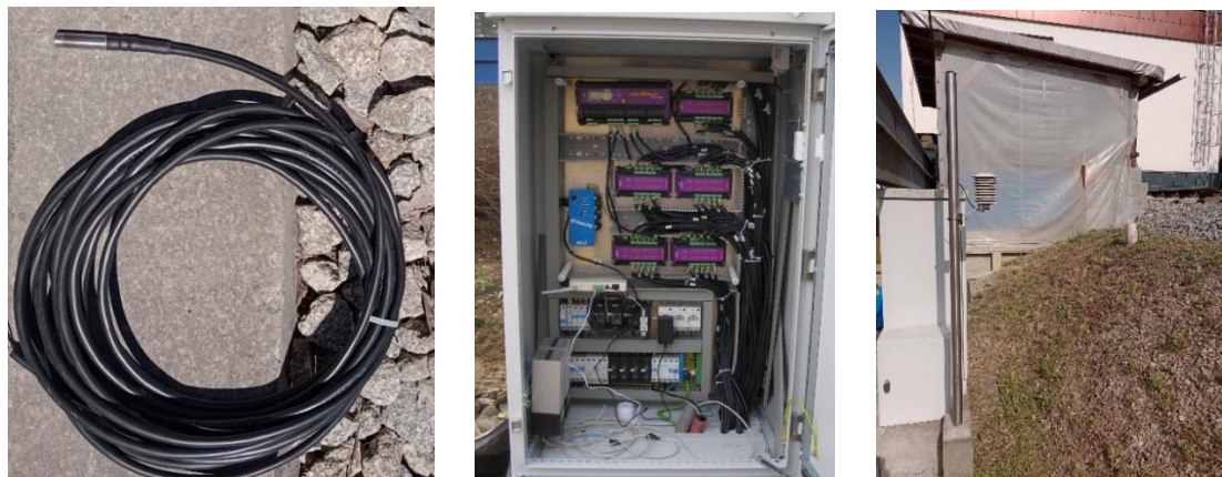
Fig. 5: Measuring equipment - Pt 1000 resistance ground temperature sensor (left), connection of the temperature sensors to the dataTaker DT80 logger via the CEM20 channel expansion modules (center), Comet T3419 sensor housed in a specialized meteorological shield (right).
