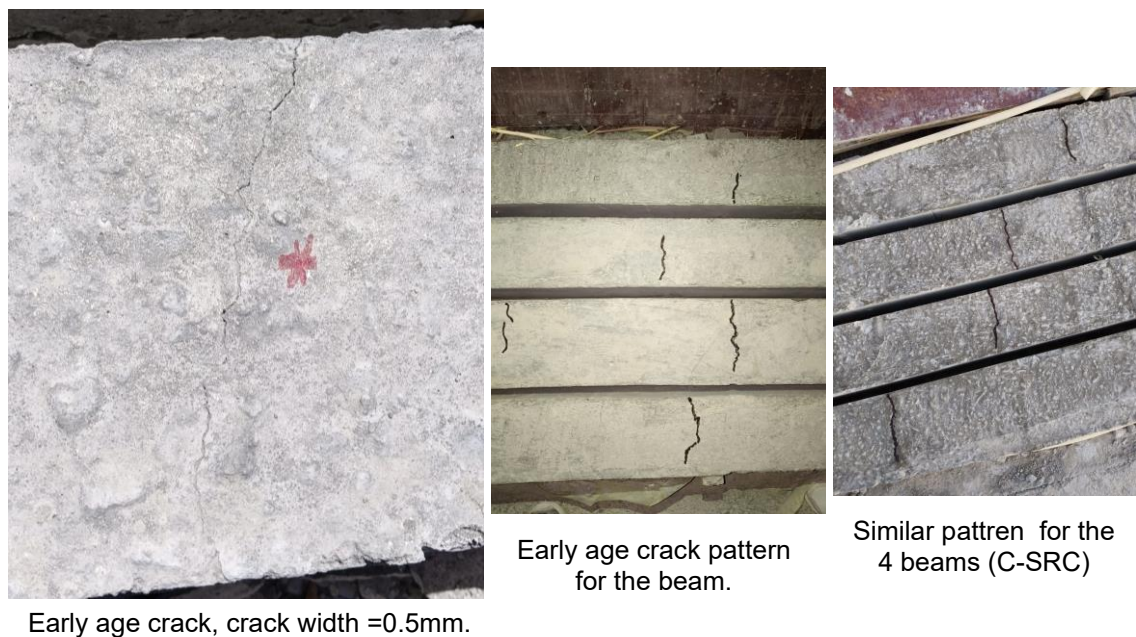
Fig. 13: Early age cracks in the tested beams.
