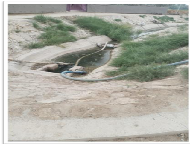
Fig. 7: The violations observed on sedimentation basin of DC 11 canal.
