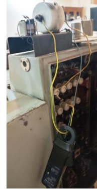
Fig. 6 – Position of the transformers and the current probe.
