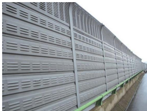
Fig. 5 – Phonoabsorbent panels made of metallic materials (Ștefan, 2018).
