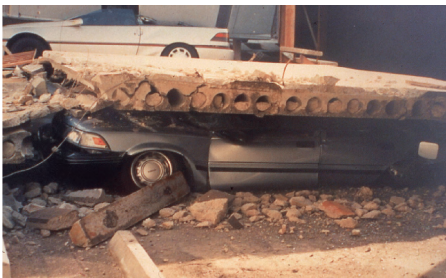
Fig. 5 – “Collapse of precast concrete hollow core floor (1994 Northridge Earthquake)” (FIB 27, 2003).
