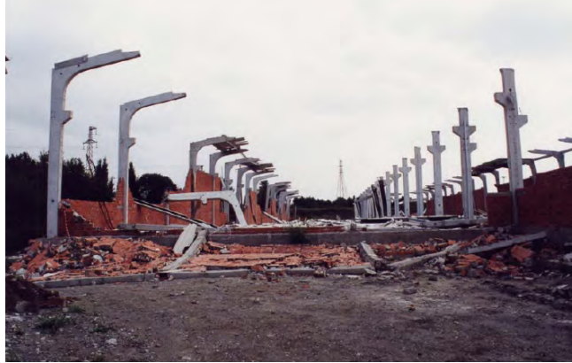
Fig. 8 – “Failure of columns due to interaction with stiff masonry infill (1999 Kocaeli Earthquake)” (FIB 27, 2003).
