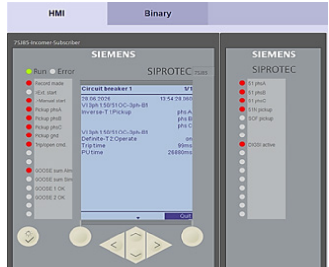
Figure 6: Relay HMI response, displaying the definite-time overcurrent protection trip and pickup time.
