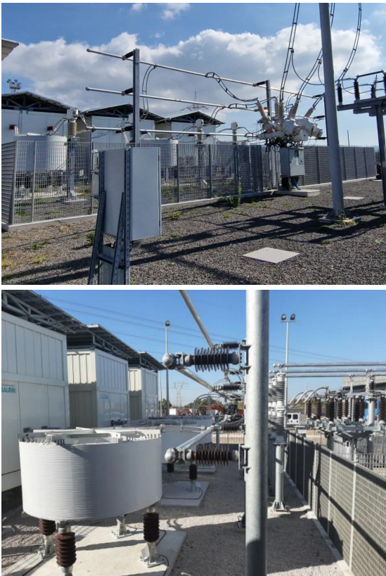
Figure 6: Terna's containerized solution for STATCOM arrangement (left side: Aurelia substation, by NIDEC, using Hybrid Switchgear; right side: Latina Substation, by SIEMENS, using air insulated switchgear)
