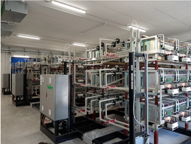
Figure 7: Terna's indoor solution for STATCOM arrangement (Galatina substation, by NIDEC)
