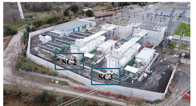
Figure 7: Top view of the SC2 and SC3 plant.
