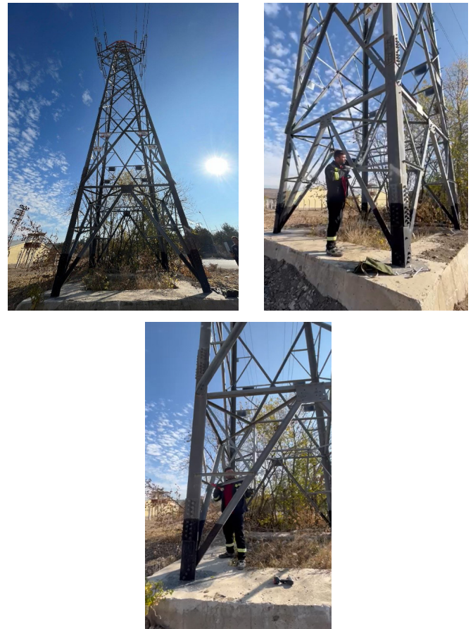
Figure 9: Controlled field test demonstrating unscrewing by screw gun and by hand on a transmission tower
