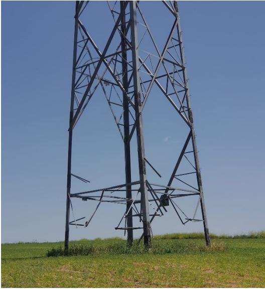
Figure 10: 154-kV transmission tower with removed iron components and structural weakening
