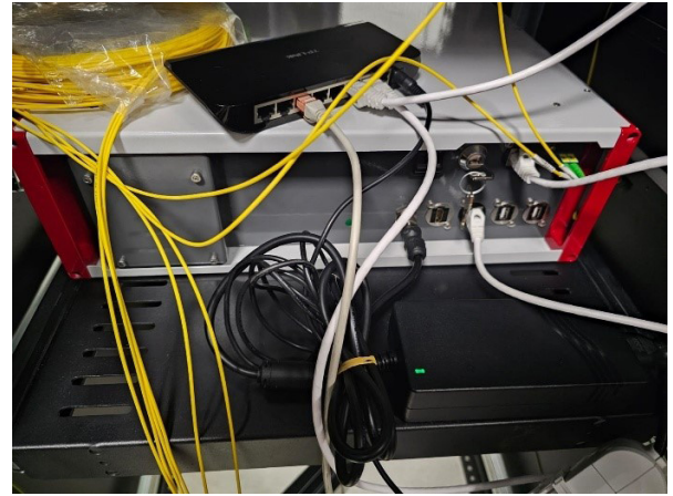
Figure 4: Installation and fiber optic connection of the DAS system within a rack cabinet
