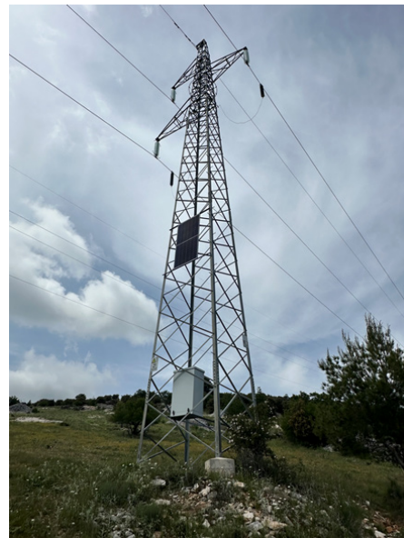
Figure 7: Lightning current monitoring system on the overhead line tower
