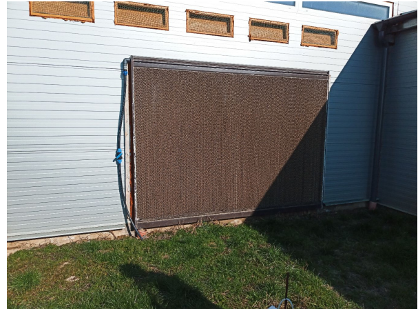
Figure 2. Air intakes and evaporative cooling panel in the building wall
