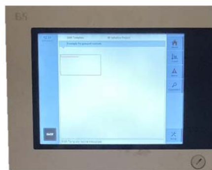
Fig. 9 B&R Power Panel 500 – HMI display, placed on the front panel of the switchboard Electrical drive – ABB 3GAA101520-ADE662
