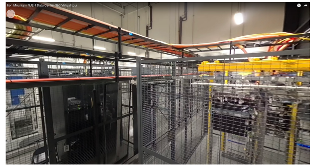
Figure 12: Screenshot from the Virtual Tour of an Iron Mountain Data Center © Iron Mountain Inc.
