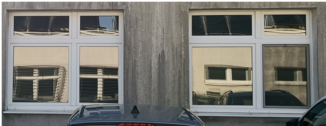
Figure 1. “Pillowing” of IGU component panes causing distortion of the reflected image.
