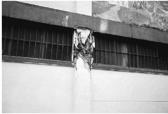
Figure 1. Short column failure due to partial infill wall, the 1999 Colombia earthquake [5].
