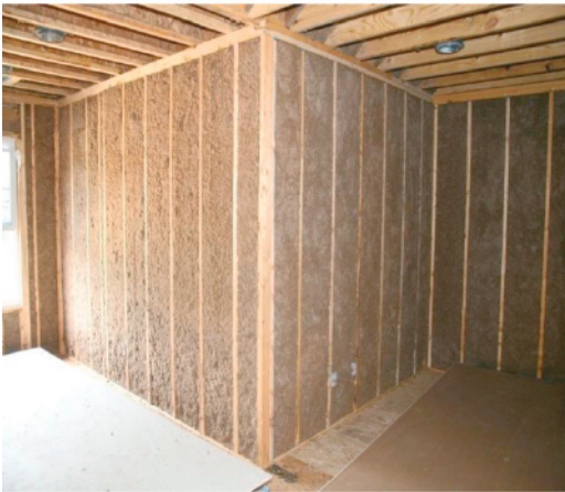
Figure 14. Cellulose thermal insulation
